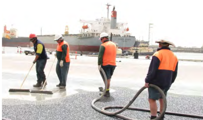
RIGIPHALT® grout is blended and applied to the pavement surface using proprietary techniques.
