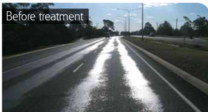
'Flushing or bleeding' is a major safety issue and cost burden for road authorities
