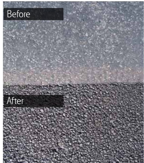
Using the UHP Watercutter to restore pavements is a long term solution for texture and skid deficient surfaces.
